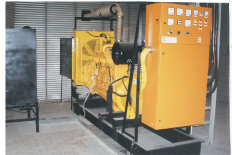
300KVA Automatic mains failure
