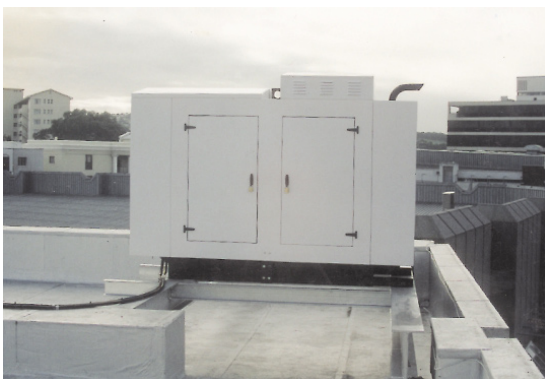
30KVA Automatic mains failure soundproof Generator Set. Standard soundproof canopy with sound levels of 65dB(A) at 7 metres in an open field.
